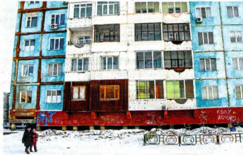
On thin ice: People passing by a cracked panel apartment in Yakutsk. Many houses here stand on stilts to ensure ventilation of the building's underbelly, and prevent it from heating the permafrost. — AFP
